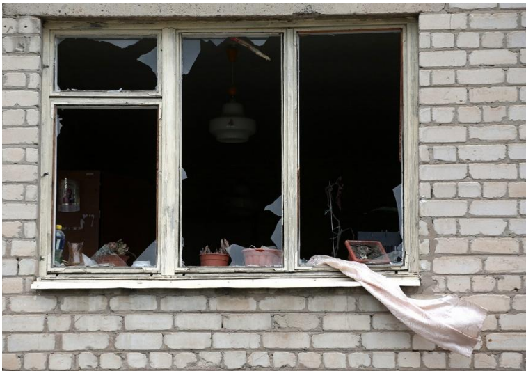
The window of a house destroyed by a missile attack in Bakhmut, Donetsk region, May 22, 2022.
