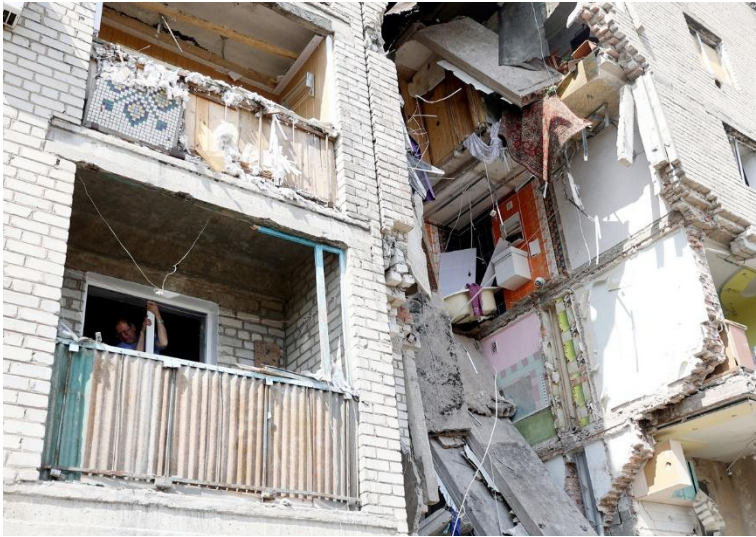
A Russian airstrike ripped apart an entire segment of an apartment building in Bakhmut, eastern Ukraine, May 20, 2022.
