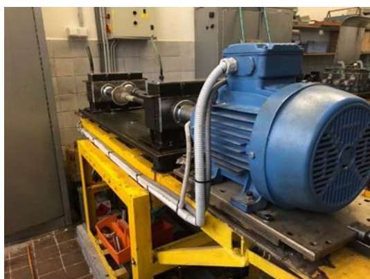
Fig. 2. Three-phase electric motor of Niemann M01
