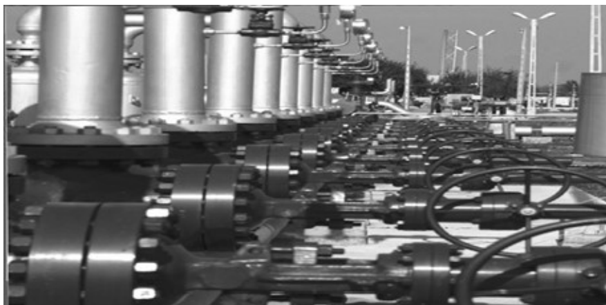
Figure 1 – The gas compression station
