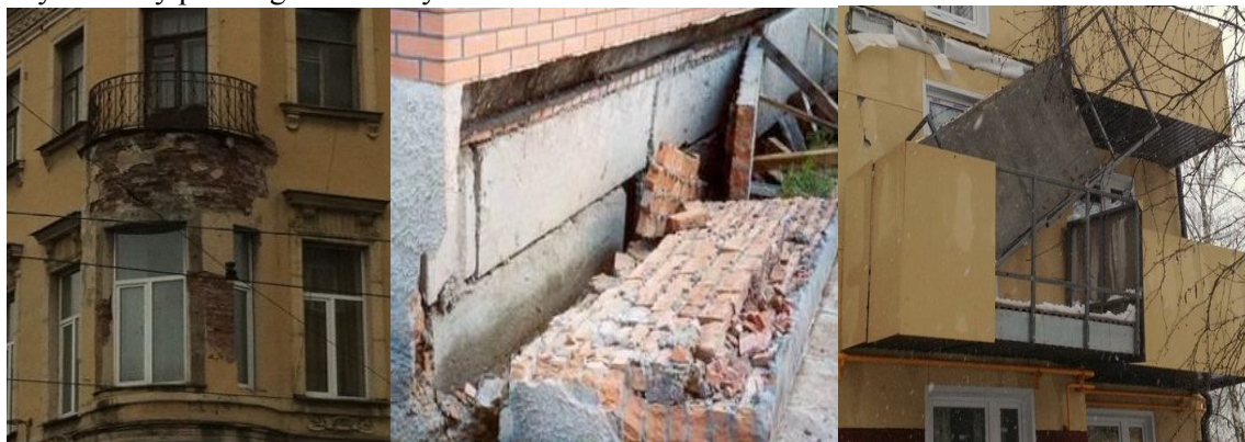
Figure 1. Inherent defects of old housing
