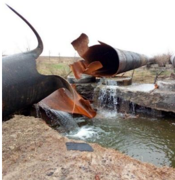
Fig. 1. Damaged water supply system “Dnipro-Mykolaiv” in the territory of the Kherson region, 2022
