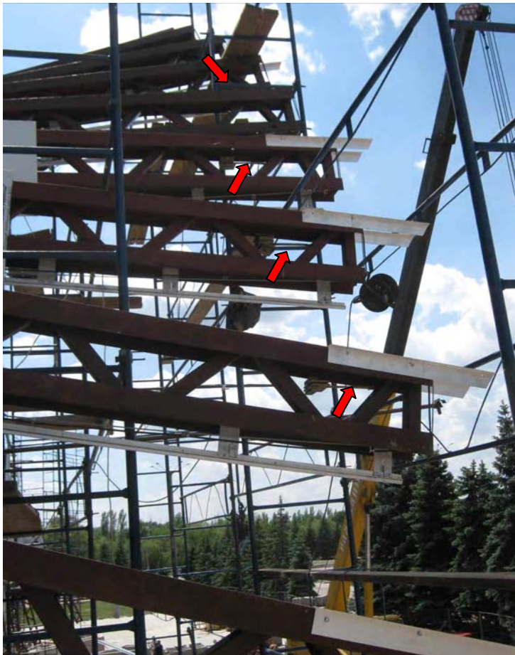
Figure 7. Realization of plate suppressors on the steel trusses of the central entrance.
