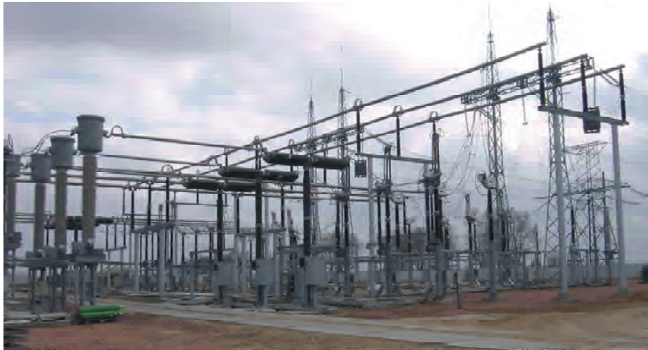
Figure 1. Rigid buses constructions of «Kievskaya» electric substation.
