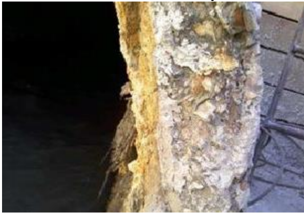
Fig. 1. Corrosion of the sewer tunnel
