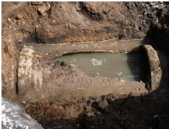
Fig. 2. Damage to the recaptured part of the collector
