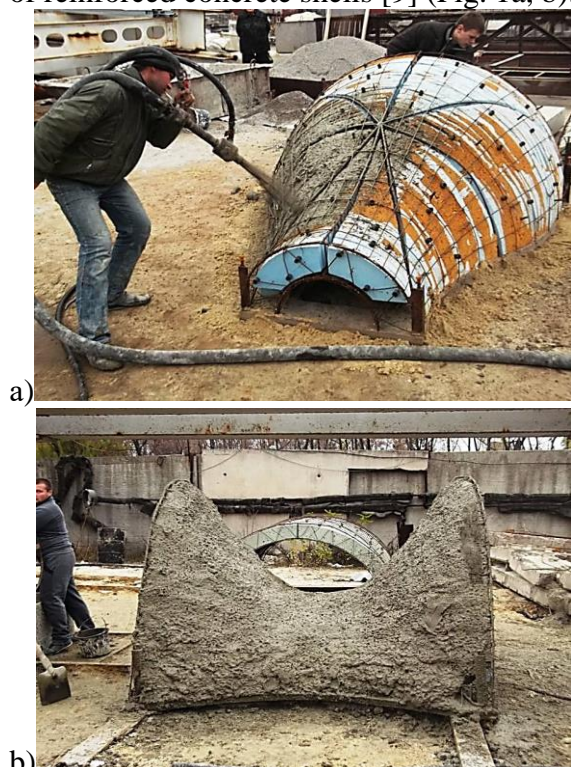
Fig. 1. Reinforced concrete casings made at construction sites by wet filling method upon off-form concreting.
