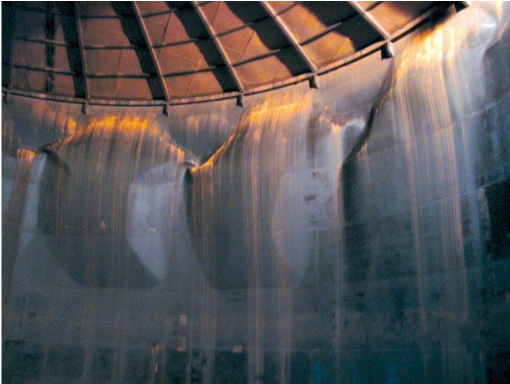
Fig. 10. Deformations of the upper part of the tank shell caused by underpressure
