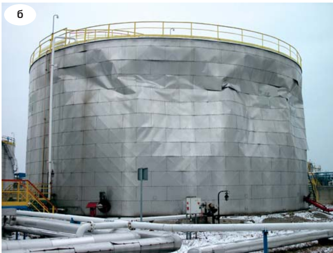
Fig. 1. Tanks injured by underpressure:
