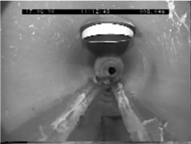
Fig. 16. The house sewer that juts out to the pipe interior
