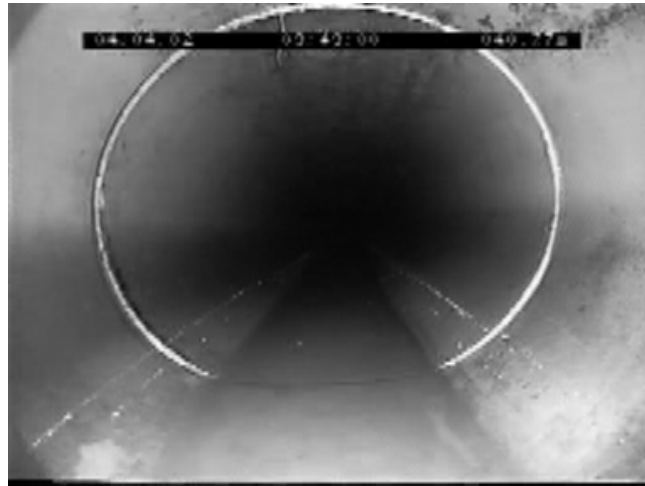
Fig.12. The deflection of the top of the pipe in the 4th class of failures
