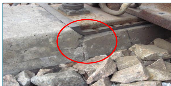
Fig. 2. Defects that arise in sleepers in the zone of geometric unevenness of the track
