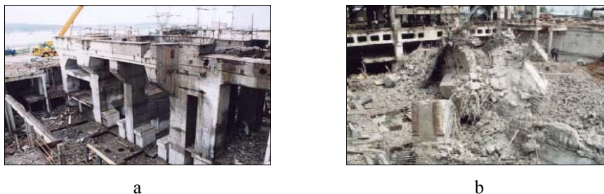
Fig. 1. An example of knocking out of concrete supported structure at Patnow power plant
