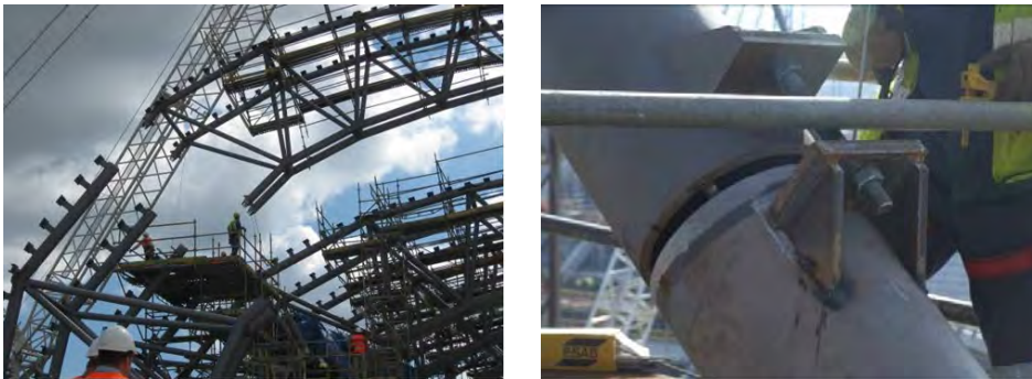
Fig. 13. The connection process of the girder roof part with the façade part
