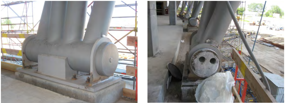
Fig. 14. Support of the girder and the place where the samples were taken
