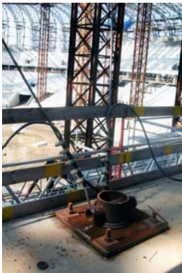
Fig. 11. Anchorage of mounting tower stays to the reinforced concrete structure of the stadium stand (stays of two neighboring towers were fastened to one anchor)
