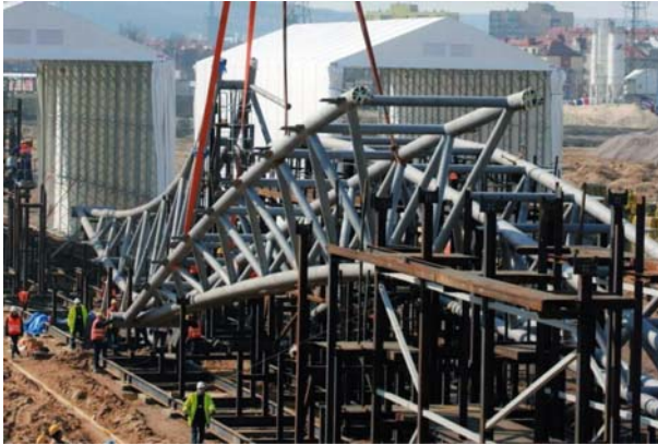
Fig. 8. Assembling of roof girders on site on two parallel assembly transoms (movable tents for protection of welding works on rainy or windy days can be seen in the background)
