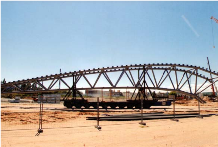
Fig. 13. A “roof” section of a roofing carrying girder (about 48 m long) transported on a self-propelled multi axle platform from the paint shop tent to the mounting crane
