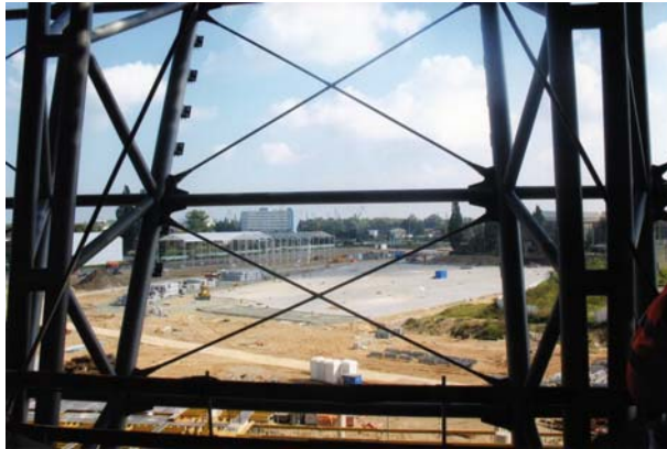
Fig. 3. Bracing between neighboring girders: ring-shaped (horizontal) made of pipes, cross braces made of circular bars
