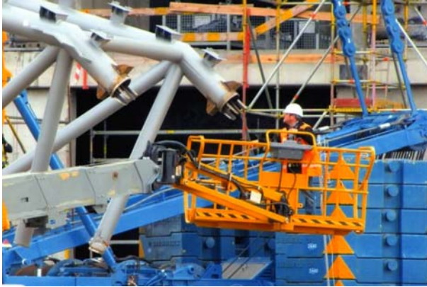
Fig. 16. Ends of the upper belt bars of a girder “roof” section fitted with fixtures to facilitate assembling
