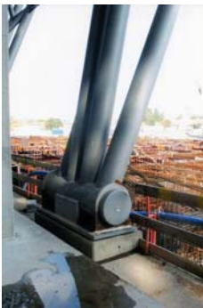
Fig. 4. Supporting of roof girders on the reinforced concrete ring in the floor at a height of about 7,0 m above ground
