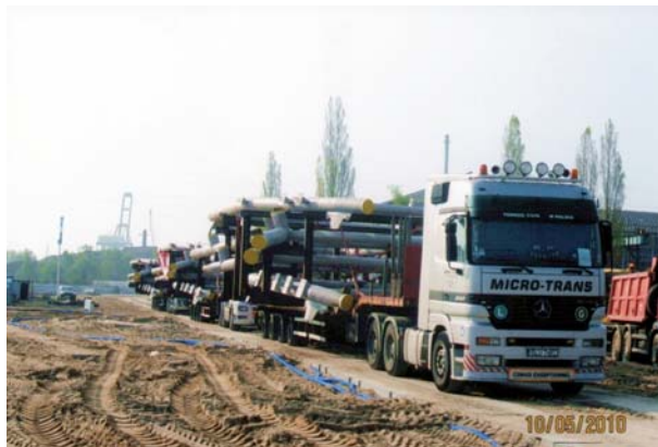
Fig. 7. Transportation of roof girder parts from the plant to the construction site (photograph courtesy of the Investor)
