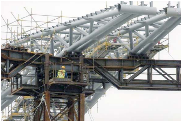
Fig. 19. Tips of two adjacent girders resting on the supporting beam. Components of the main linking ring measuring \phi 500 \times 20 mm can be seen on the girder tips
