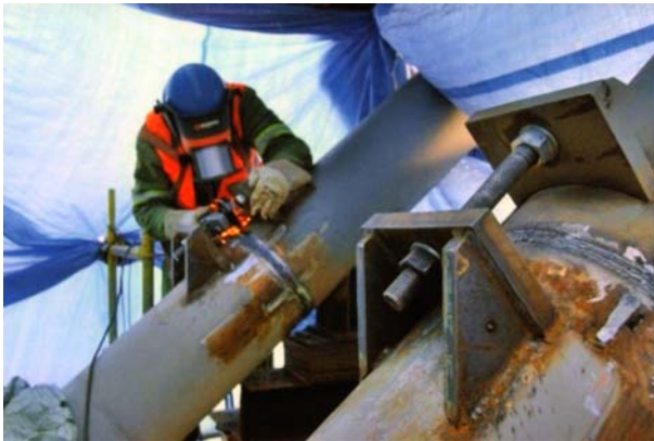
Fig. 17. Accessories for adjustment of the weld groove width of the girder upper belt pipe joint
