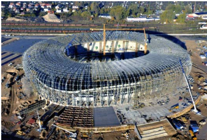
Fig. 21. Completely assembled roof carrying steel structure of the stadium (31.08.2010 – photograph courtesy of the Investor)
