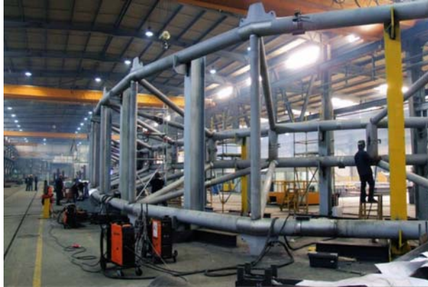
Fig. 6. Trial assembly of a three-dimensional roof girder at the plant in Gliwice (photograph courtesy of the Investor)
