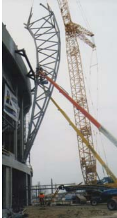
Fig. 9. The first assembled “façade” part of a roof girder (02.04.2010). The instant of temporary fastening of the girder to the segmented steel ring on the reinforced concrete stand crown beam
