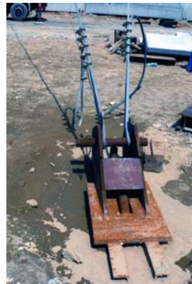
Fig. 12. Anchorage of mounting tower stays within the stadium pitch – a ground anchor (note as for Fig. 11)
