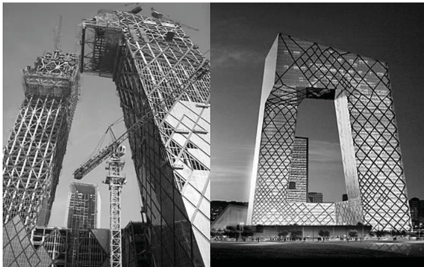
Figure 9 – View on CCTV Tower under construction (left) and the façade design of completed building (right)
