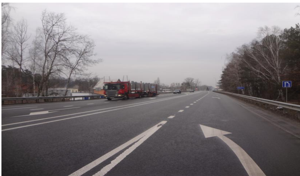
Figure 2 – Pavement condition on road Kiev – Kovel (km 33+100 , Vorzel)
