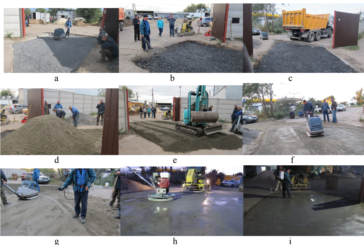
Fig. 4. Compacting of cement-concrete mixture using technology of roller-compacted cement-concrete in the experimental section: a-i – sequence of technological operations
