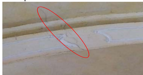
Fig. 4. The crack in ceiling
