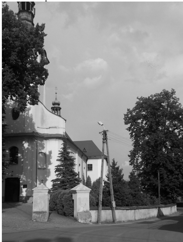
Fig. 3. Church in Rudzica - the object of restoration works protected by wireless sensor network with random access
