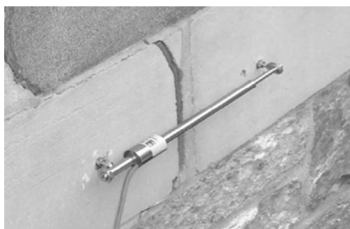
Fig. 5. Sensor for recording movements of cracked parts of the wall
