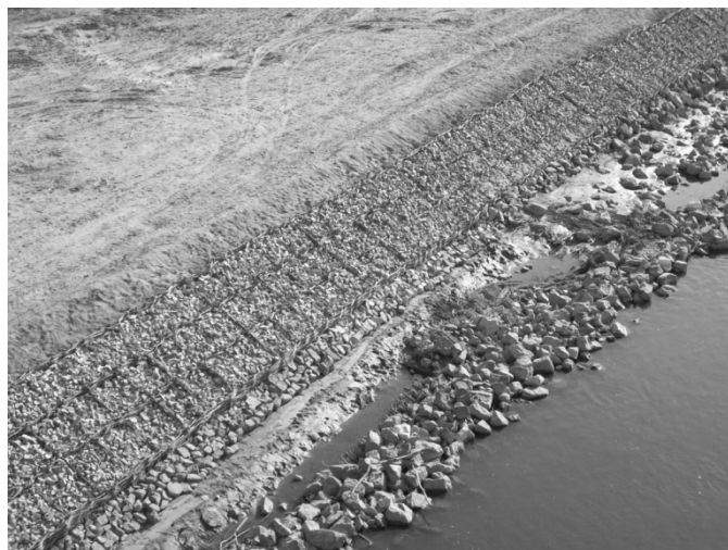
Phot. 2 – The Example of Stone and Fascine Dam on the Vistula Bank Source: From the author's private archives.
