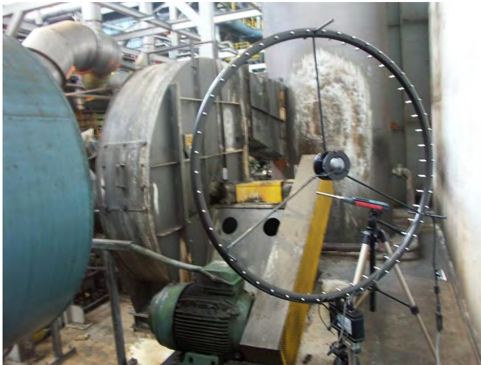
Fig. 6 Installed acoustic camera by exhaust plant
