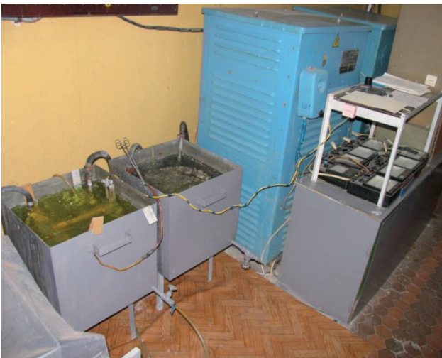
Figure 6. General view of installation for PEO
