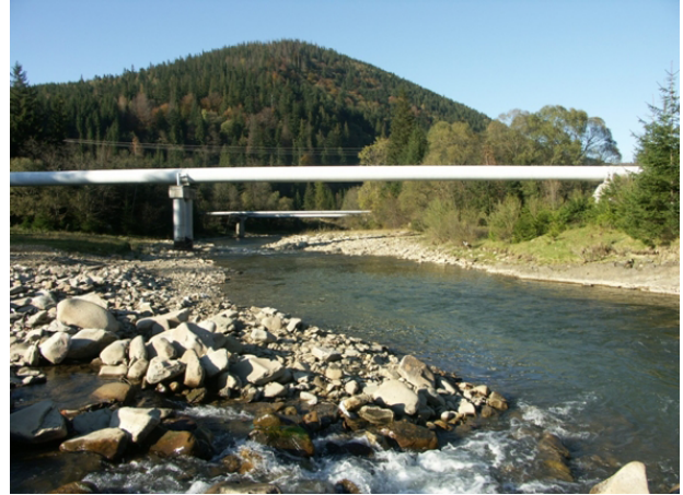
Figure 3. Pipelines passing in one technological corridor and cross natural obstacles
