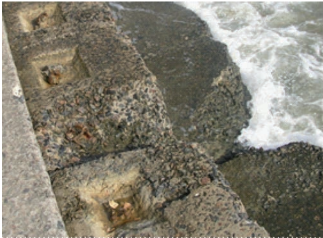
Fig. 4. Local fracture of concrete caused by local ice pressure
