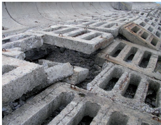
Fig. 1. The current technical condition of the coastal protection structures of the passive type on the Odessa coast (B. Fontansky cape)
