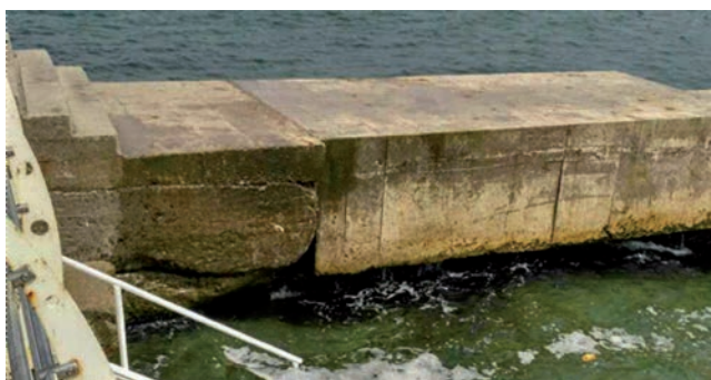
Fig. 2. The state of the root part of the buna in the zone of the variable water horizon
