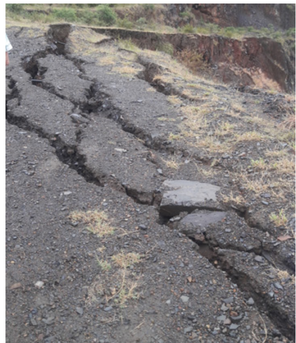
Figure 11. Visible cracks in the Southern Slopes above the Mine
