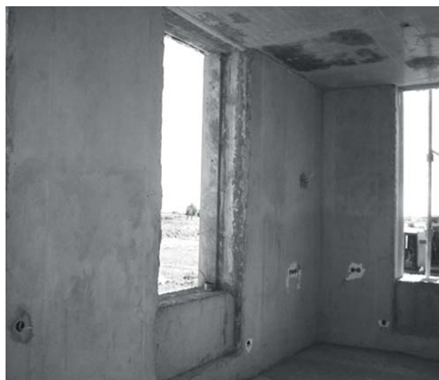
Figure 2. Detail of the interior of a residential two-storey house erected using aerated concrete wall panels
