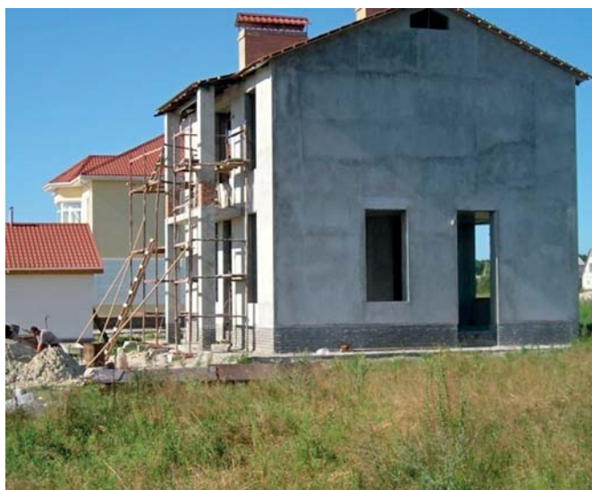
Figure 1. Residential two-storey house, erected with the use of aerated concrete wall panels
