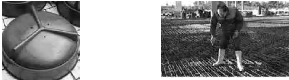
Figure 5. Control of filling lower zone of slabs with voids in the form of inverted caps with concrete mixture.
