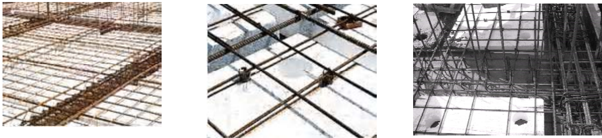
Figure 8. Flat slabs with inserts in the form of rectangular expanded polystyrene prisms.
