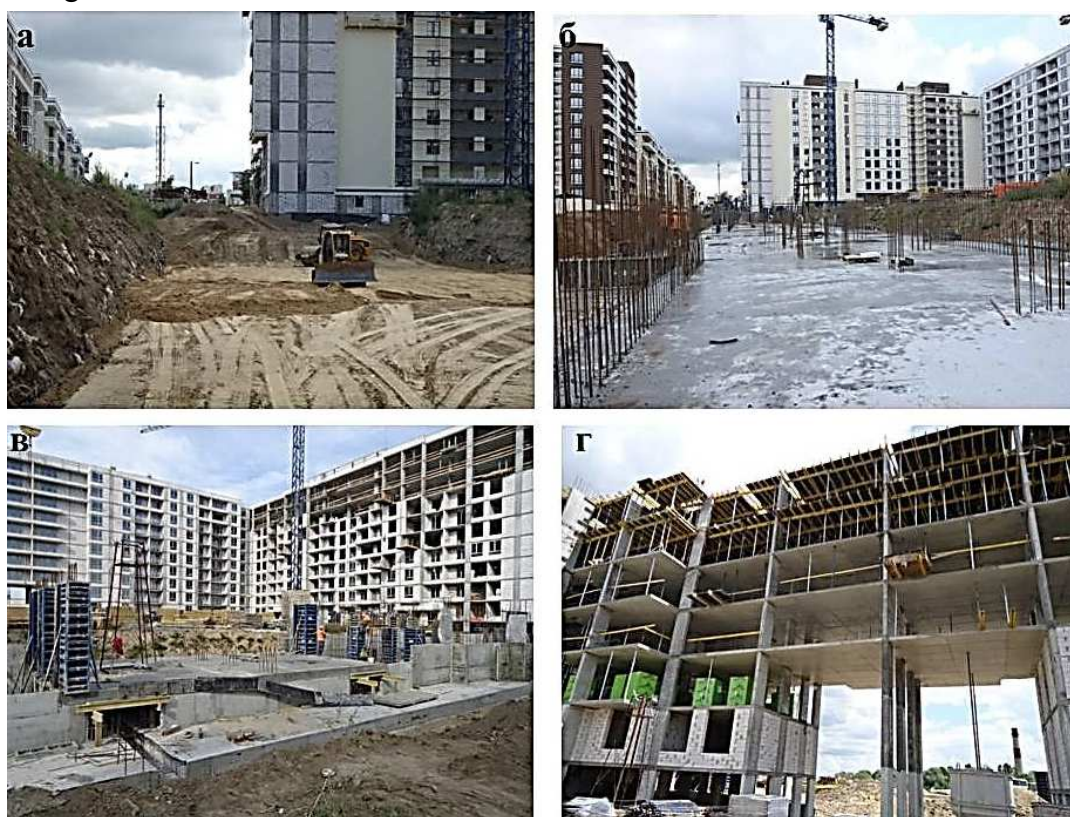
Fig. 6. General view performance of work: preparation of foundation (a); the device of the foundation slab (b); the device of basement (c); building frame (d)
