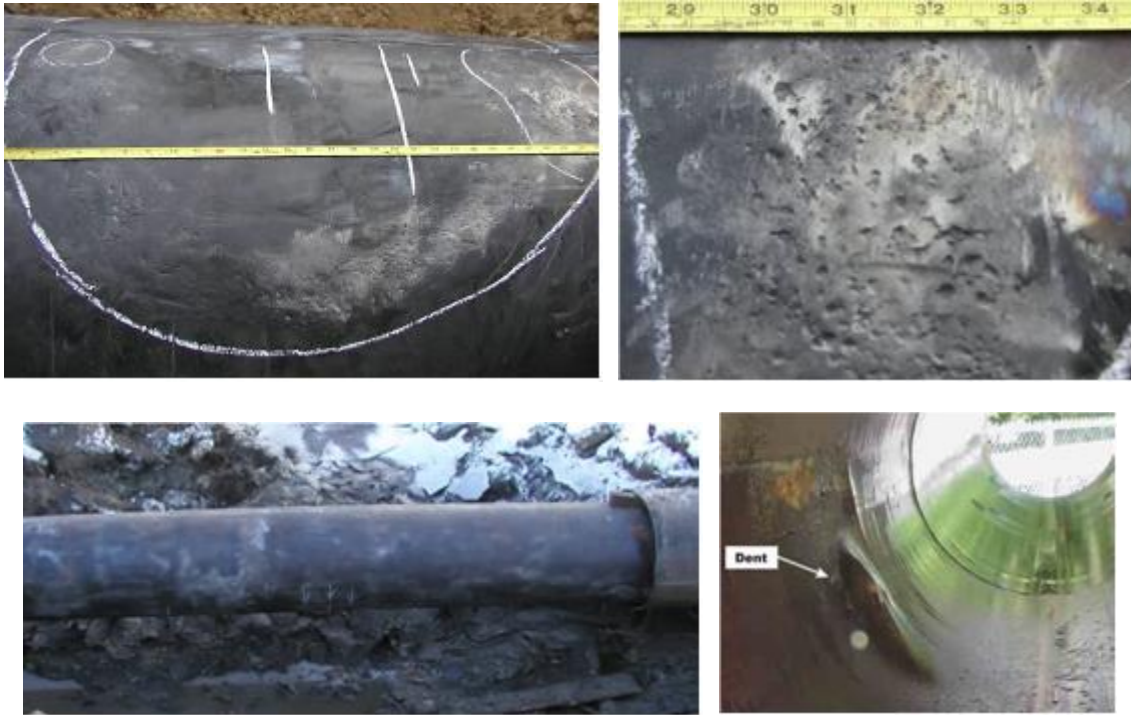
Figure 3. Examples of pipeline walls deformation
