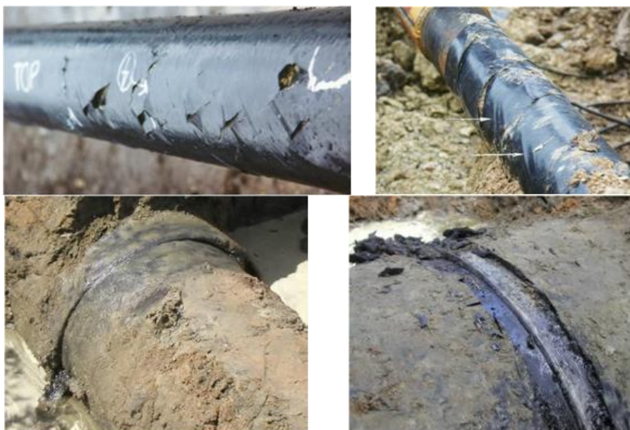
Figure 5. Examples of pipeline coating damages
