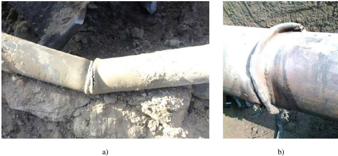
Figure 2. Examples gas pipeline failure in the surface subsidence trough: a) – DN100; b) – DN300
