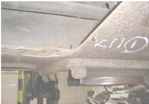
Fig. 5. The crack on the welding seam at the joint of the lower sheet of span bolster with the longitudinal tie rod
