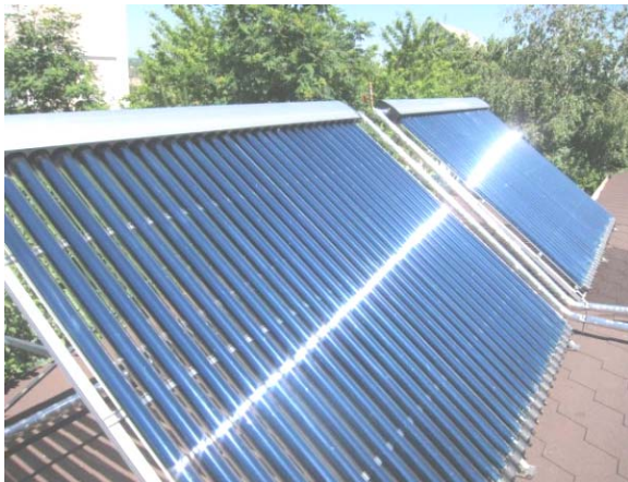
Fig. 11. Solar collector on the building roof
