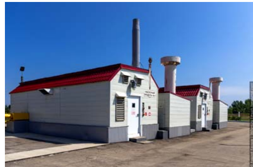
Fig. 3. Buildings with ammonia pumps
